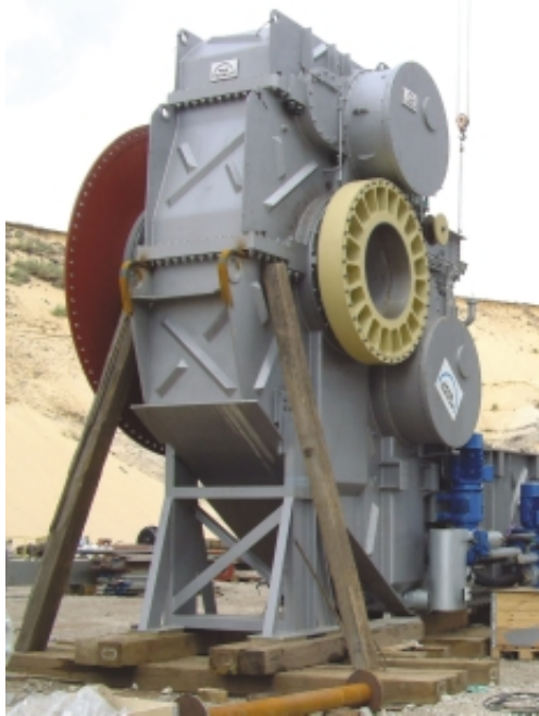
Figure 1: 80 ton gear on the main drive of the bucket wheel
